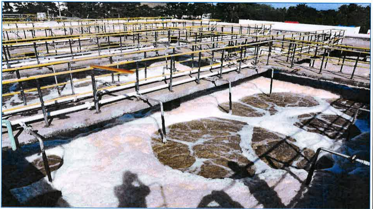
Biological Treatment plant
