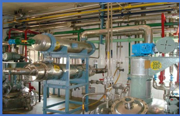
Vent condensers for VOC control
